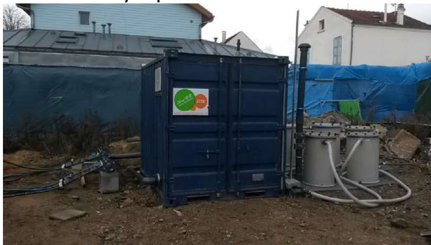
Photograph of SVE treatment facilities
