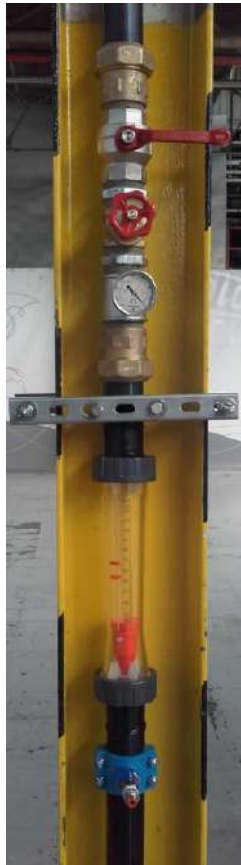
Examples of instruments along each extraction line
