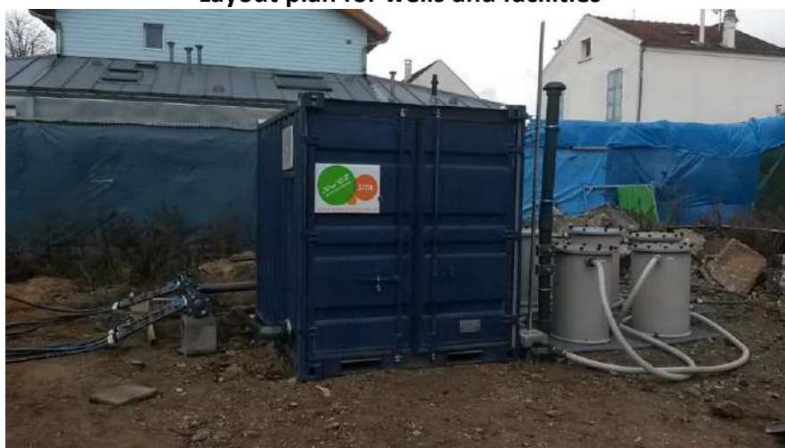
Photograph of SVE treatment facilities
