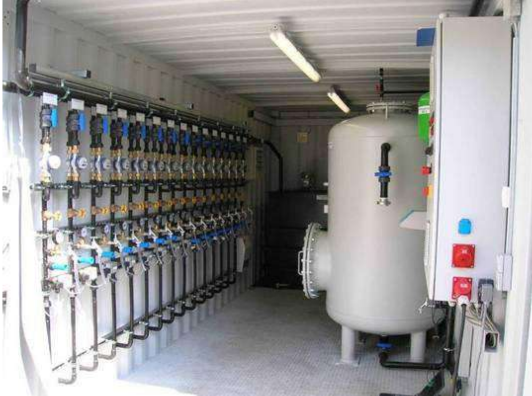
ISCO plant technology
