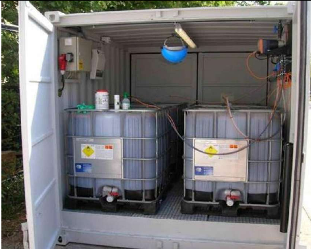
ISCO dosing station
