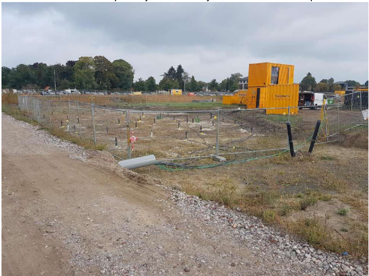
Overview injection filters in source zone
