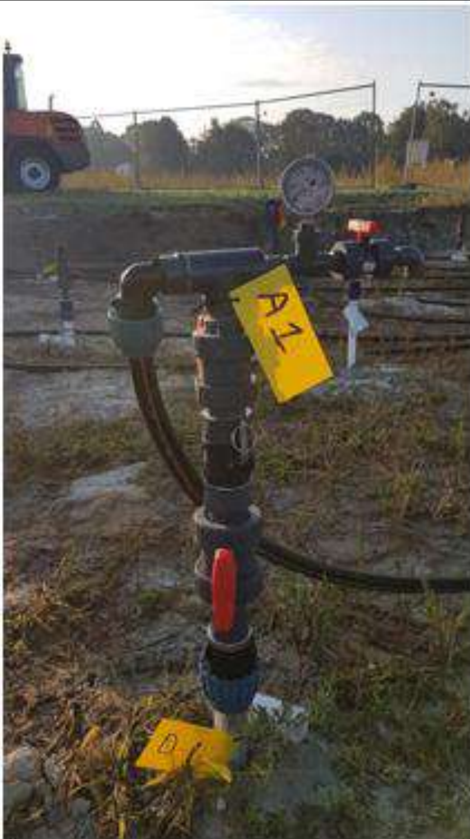
Detail injection well manifold
