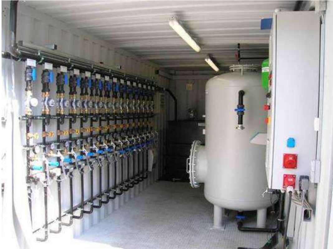
ISCO plant technology
