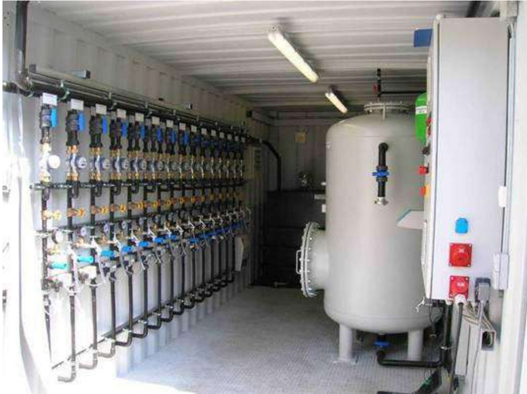
ISCO plant technology
