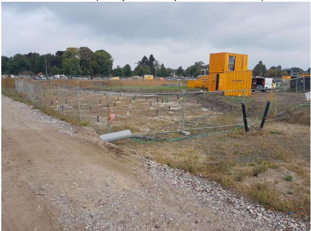
Overview injection filters in source zone
