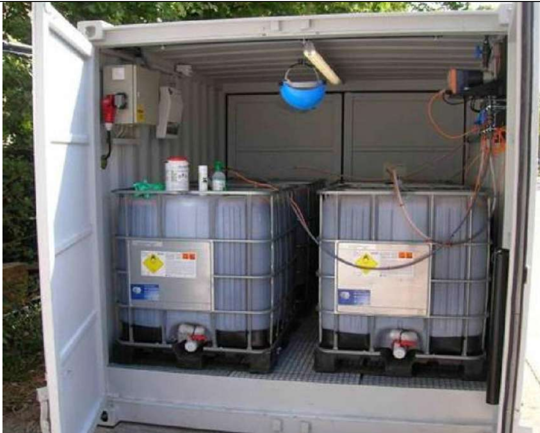
ISCO dosing station
