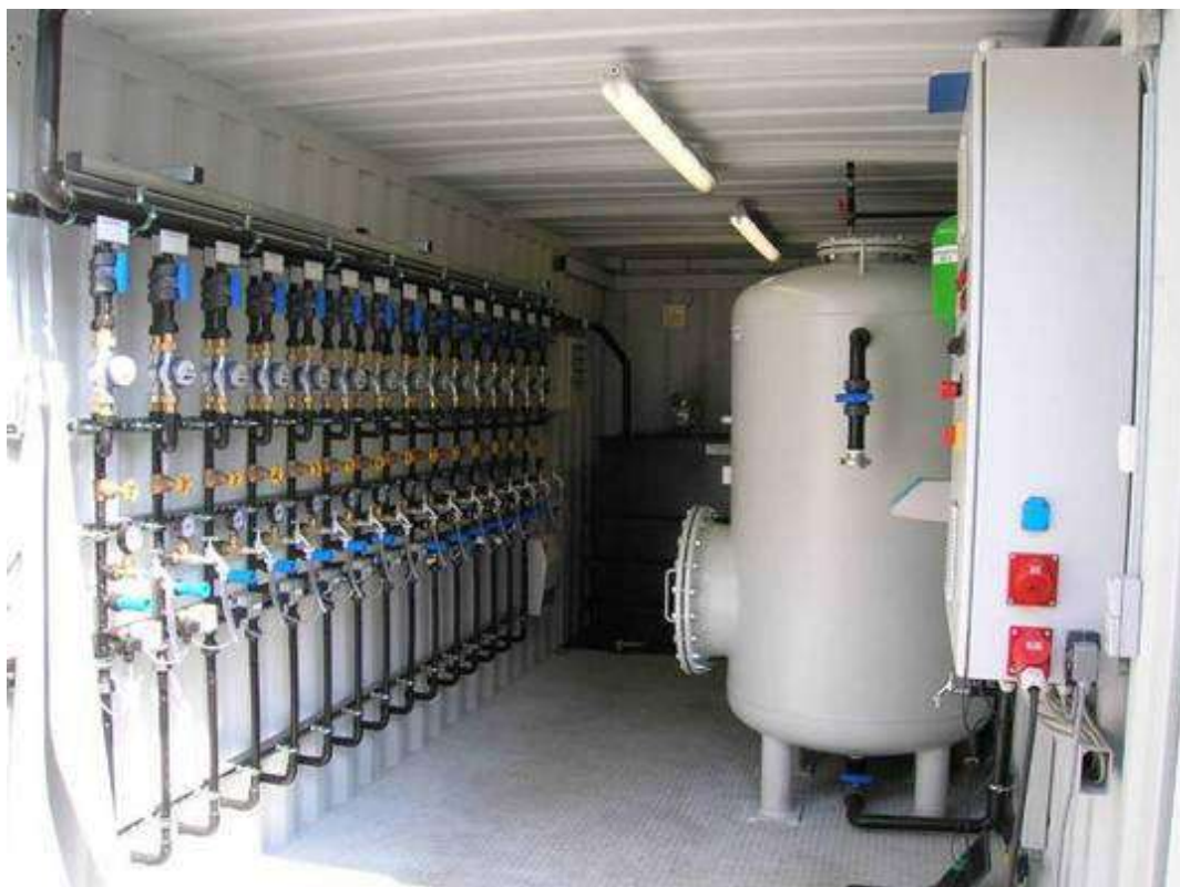
ISCO plant technology
