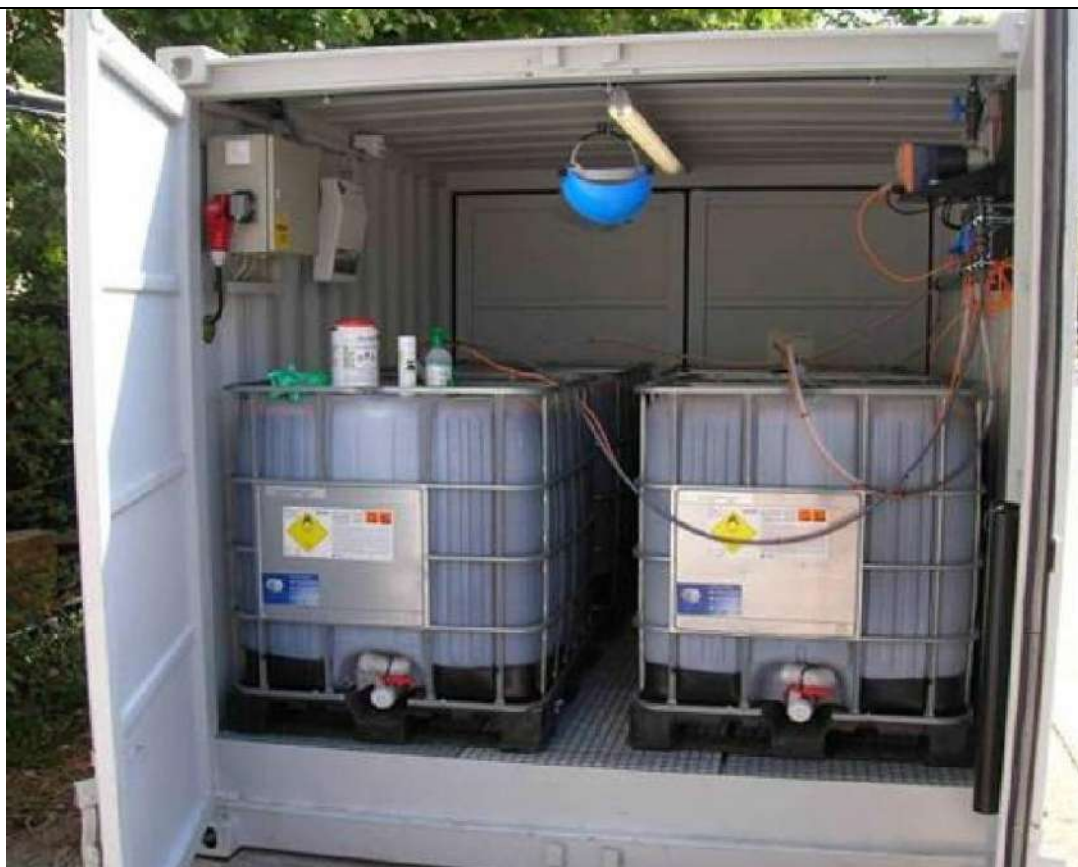
ISCO dosing station
