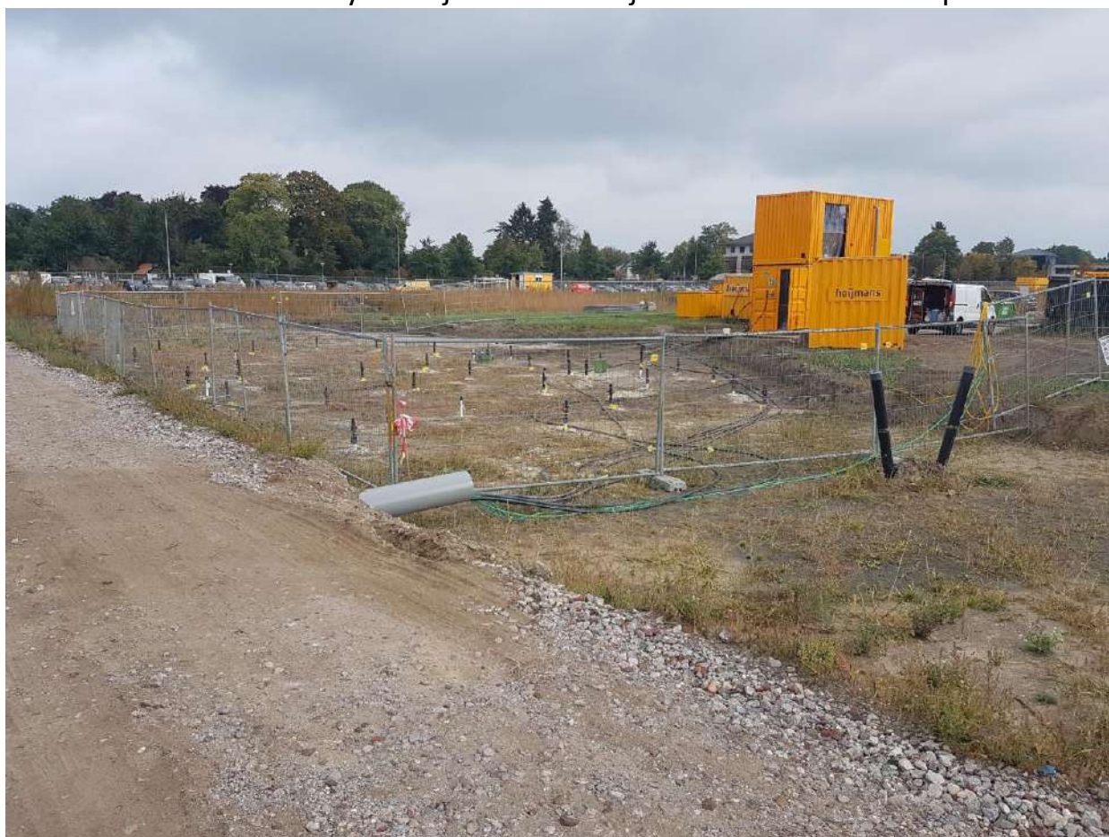
Overview injection filters in source zone
