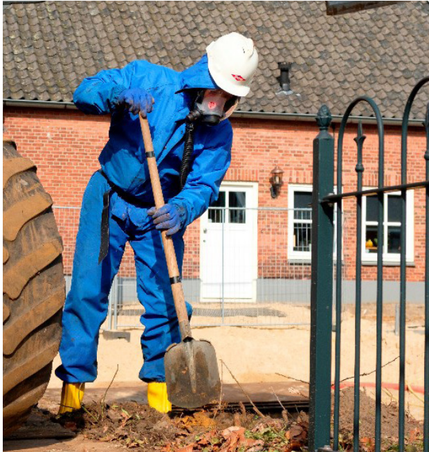
Visual detection of asbestos during remediation | NTP
